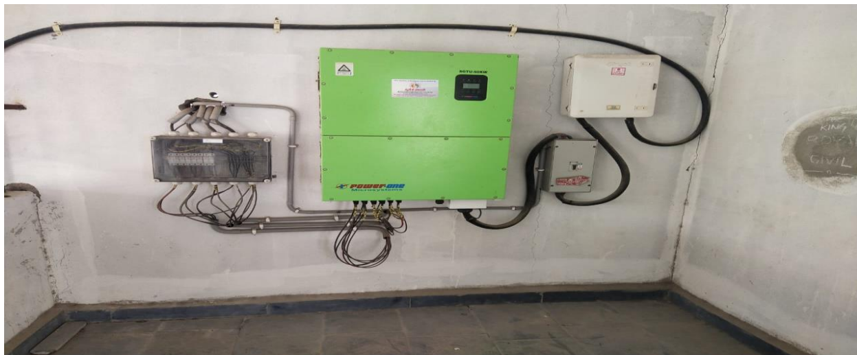
Wheeling to GRID connection
