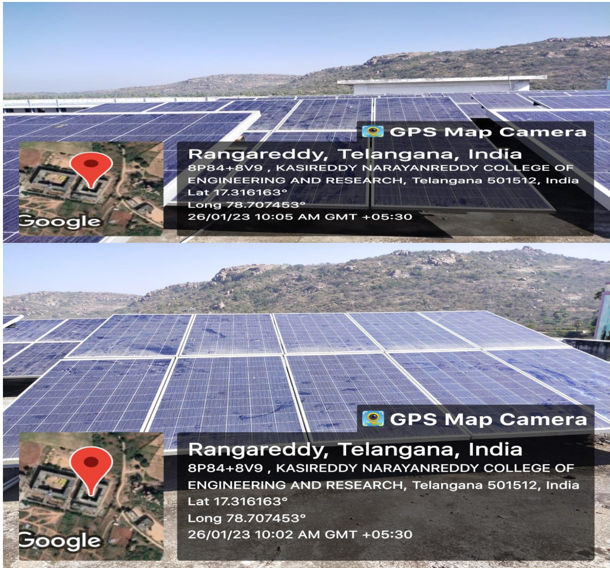
View of Solar Power plant 75 KWp.
